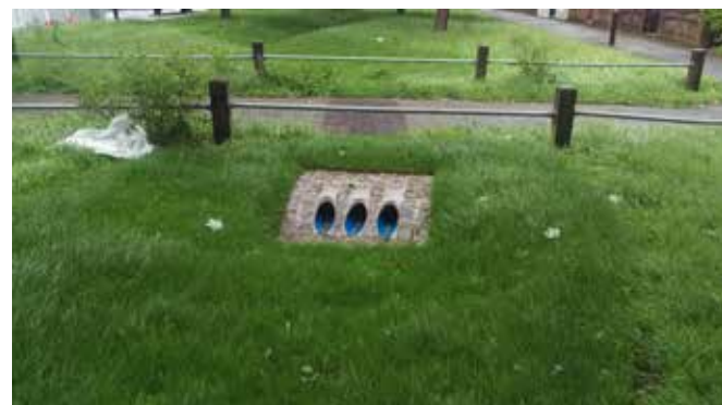
Concrete pipe surround has been used here to provide minimal cover for a driveway crossing at Devonshire Hill, Haringey.
