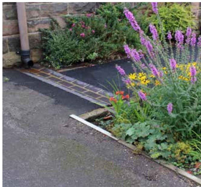
Strutts Centre, Belper. A retrofit downpipe shoe and brick channel into a raingarden.
